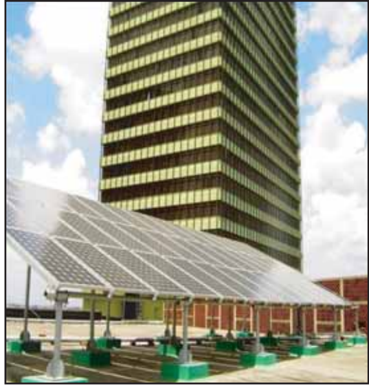
Solar panel on Bangladesh Bank rooftop
